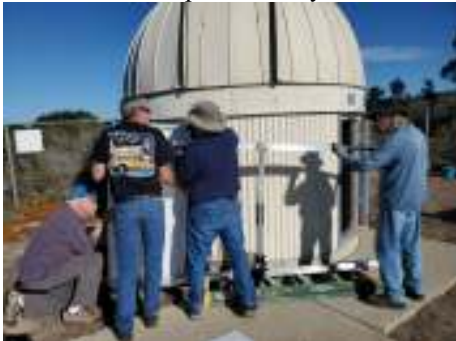
Setup Solar array
